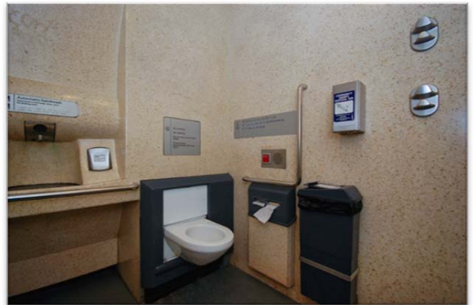
Wall mounted contaminated sharps container
